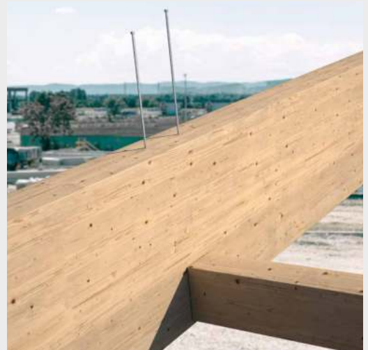
Reinforcement orthogonal to grain for hanging load due to joining of main-secondary beams.
